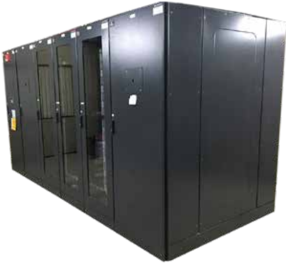
Green Edge Data Center at Rail Nilayam, S.C.Railway, Secunderabad.
