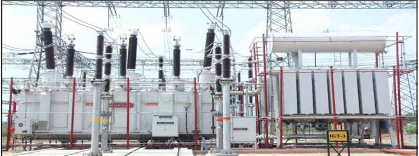
500 MVA 400/220/33 KV POWER TRANSFORMER
