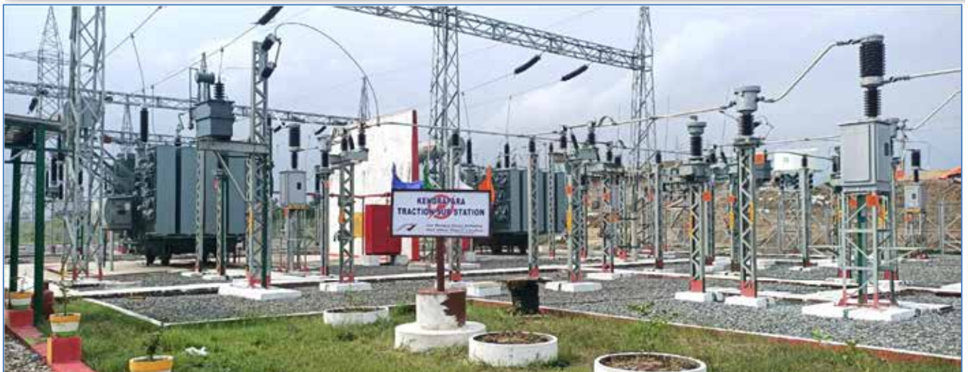
132/27 KV TRACTION SUB-STATION (TSS)
