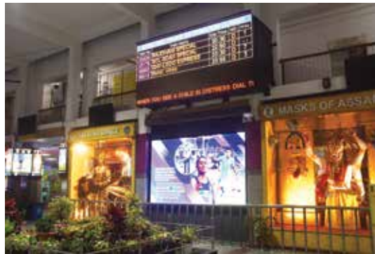
Integrated Passenger Information System provided at Guwahati Railway Station
